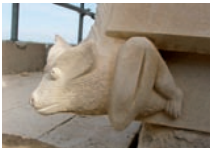
Details of the buttress repairs at Moulton, simply fixed with mortar joints and stainless steel dowels between blocks, and interlocked with the existing stonework behind to prevent it toppling forward (Photos: Katie Worthington, by courtesy of CEL Ltd)
