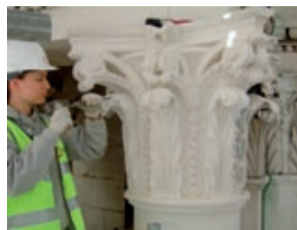
Top, detail showing the horizontal notch at the back of the opening and, middle, the new stone fixed in position pending carving, below (Photos: Katie Worthington by courtesy of Stonewest Ltd)
