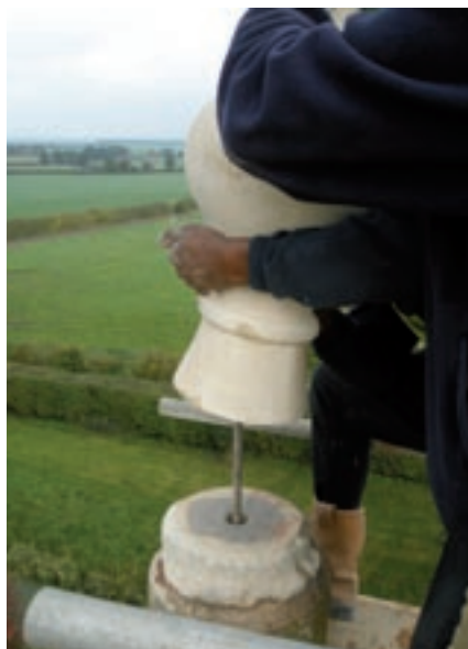
Lowering a heavy stone finial onto a dowel (Photo: Katie Worthington, by courtesy of CEL Ltd)
