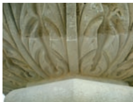
An indent repair at the Royal Pavilion, Brighton, showing the hole in the underside of one of the palm leafed capitals after cutting out the damaged section (left) and the repair (right). The detail (below) of the work before pointing shows more clearly that the lines of the new work copy the lines of the original carving, and are slightly proud of the weathered surface above.
