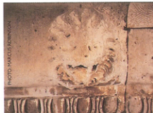
Some of the carving was too badly weathered to be saved and was replaced.
